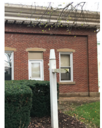
overgrown landscaping and unused signpost
