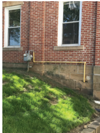
two-toned, street facing gas meter
