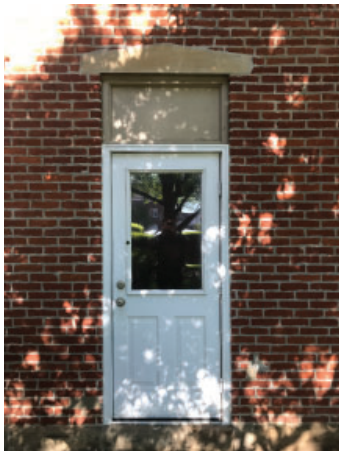
inappropriate replacement doors - painted transoms
