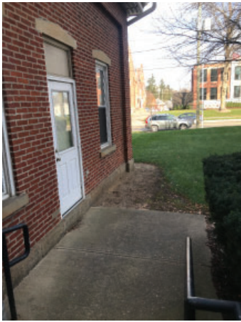
does not meet ADA
