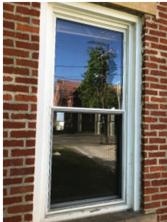
inappropriate vinyl replacement windows
