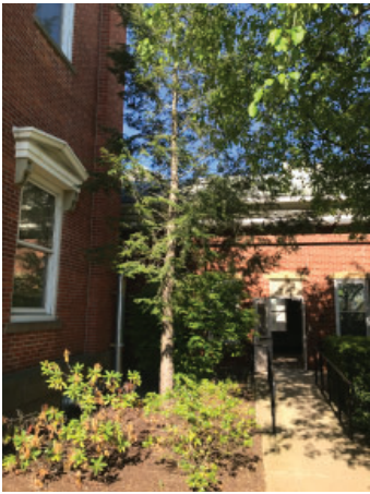
scrub tree too close to building foundation
