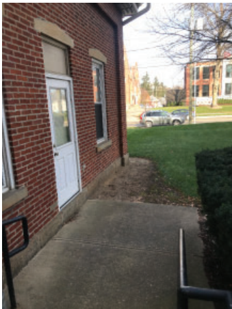
does not meet ADA
