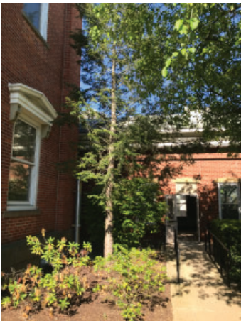
scrub tree too close to building foundation
