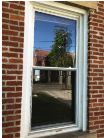
inappropriate vinyl replacement windows
