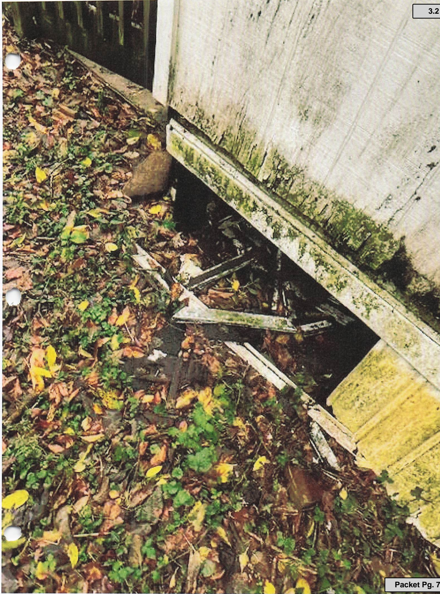
Communication: 305 W Pleasant Condemnation Proposal BPMA PT II 12.02.25 (Property Maintenance Appeal - Proposal of Condemnation)
