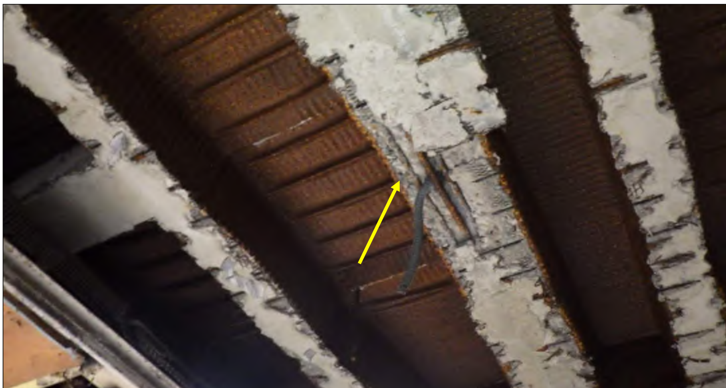
Photo 46: Exposed corroded internal steel reinforcement at a joist (arrow).
