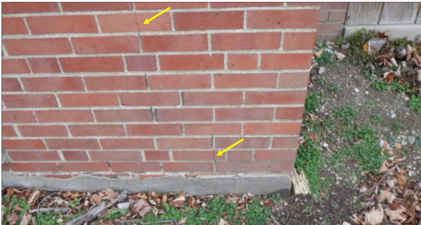
Photo 29: Hairline vertical cracking through brick masonry near base of wall.
