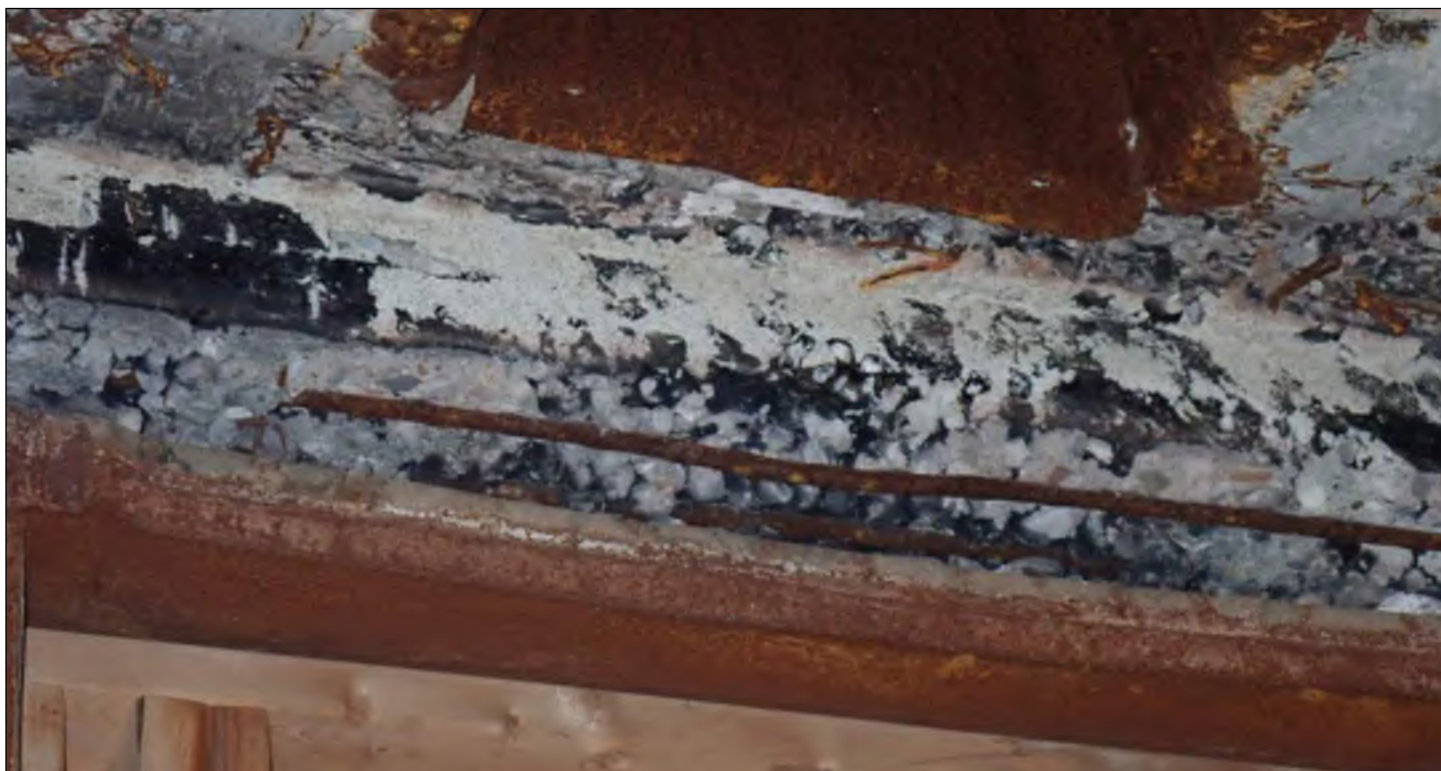
Photo 50: Close-up view of exposed corroded reinforcement at a lintel.
