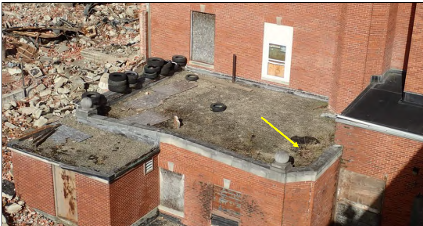
Photo 16: Overall view of boiler room roof, looking north. Note vegetation growth (arrow).
