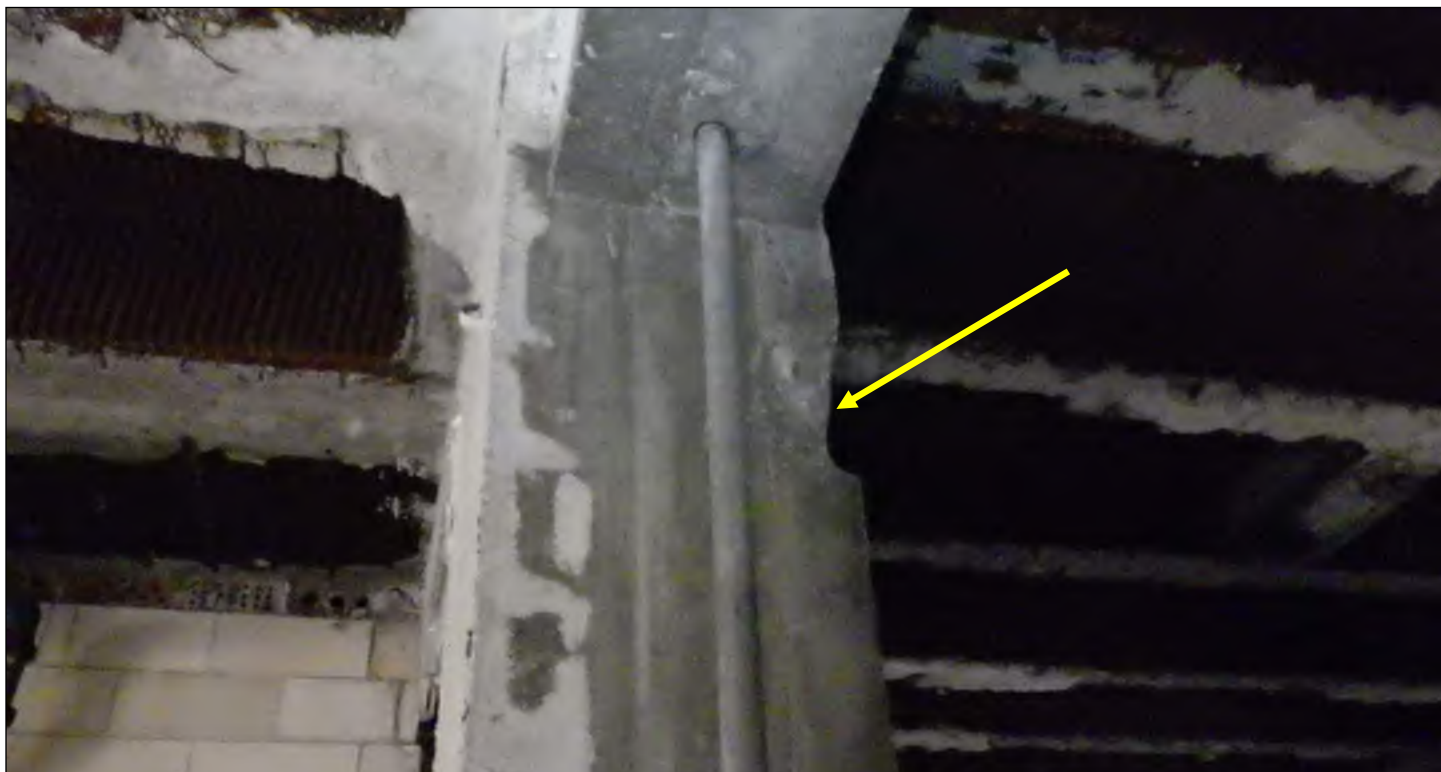
Photo 57: Missing chunk of concrete from the corner of a column (arrow).
