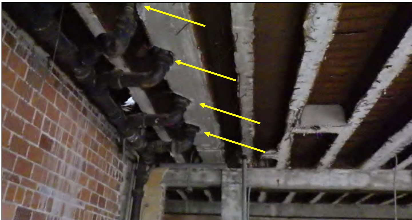
Photo 52: Piping penetrations in a double-width concrete joist (arrows).
