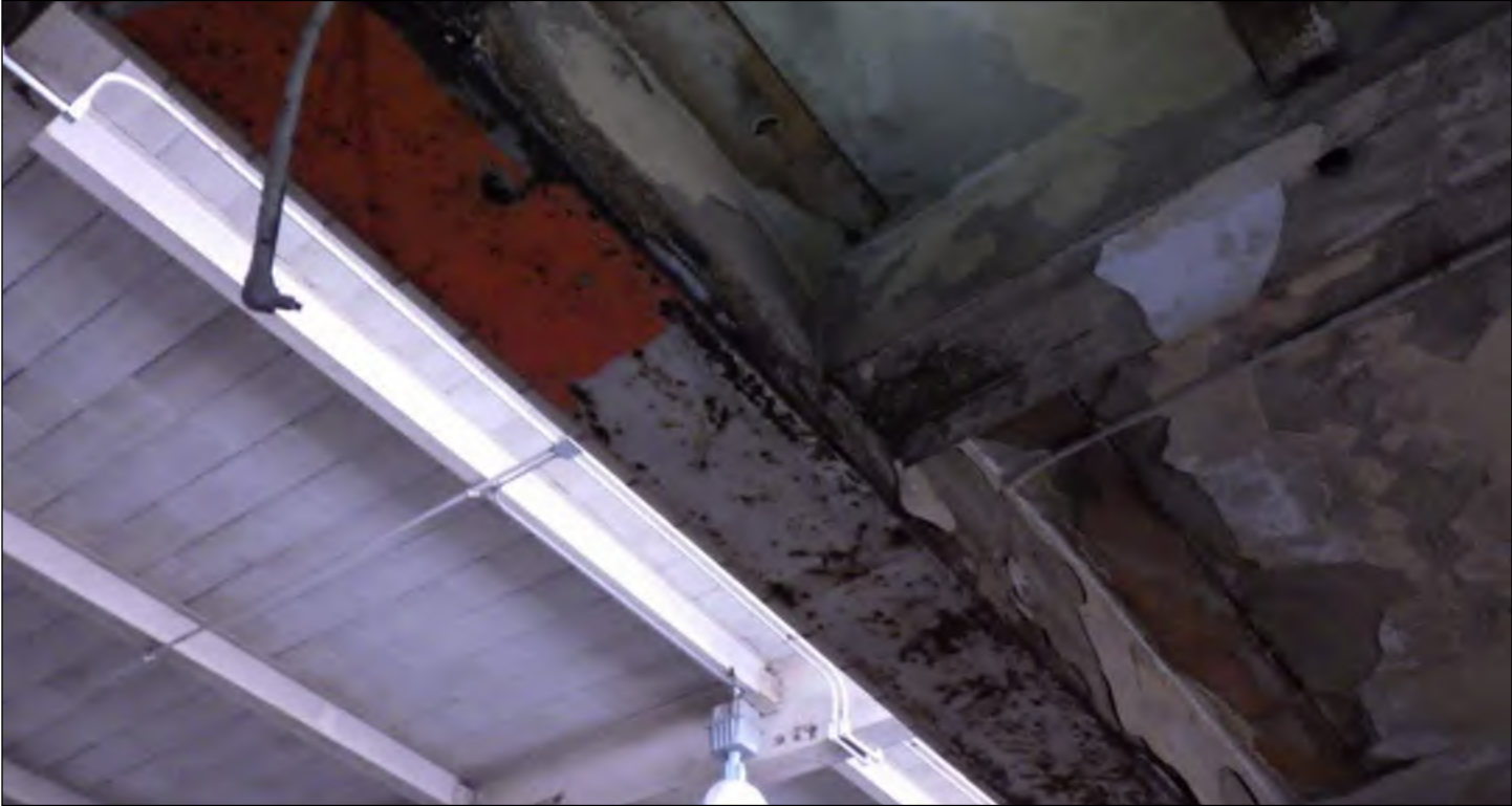
Photo 63: Corrosion (rust) at the underside of large steel beam at west side of gymnasium roof.
