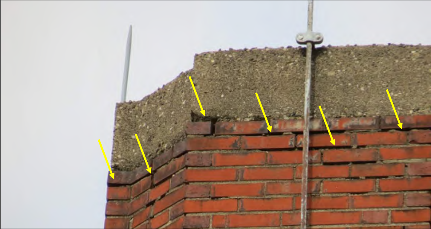
Photo 21: Mortar joint deterioration near smokestack crown.
