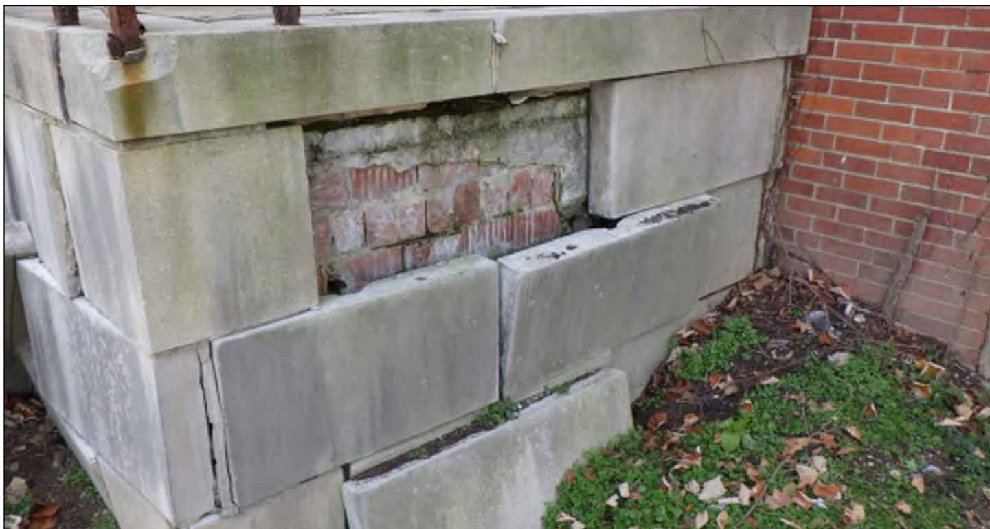
Photo 36: Bricks with missing mortar at exterior stairs by east entrance.
