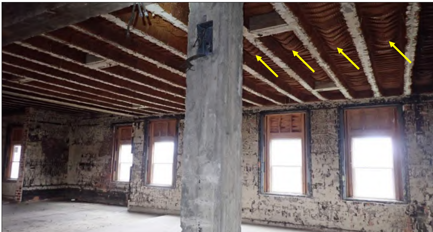
Photo 41: Overall view of reinforced concrete joists with leave-in-place metal tile formwork. Note construction anomalies (arrows).
