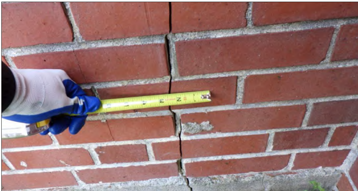
Photo 27: Vertical crack near base of brick masonry bearing wall.
