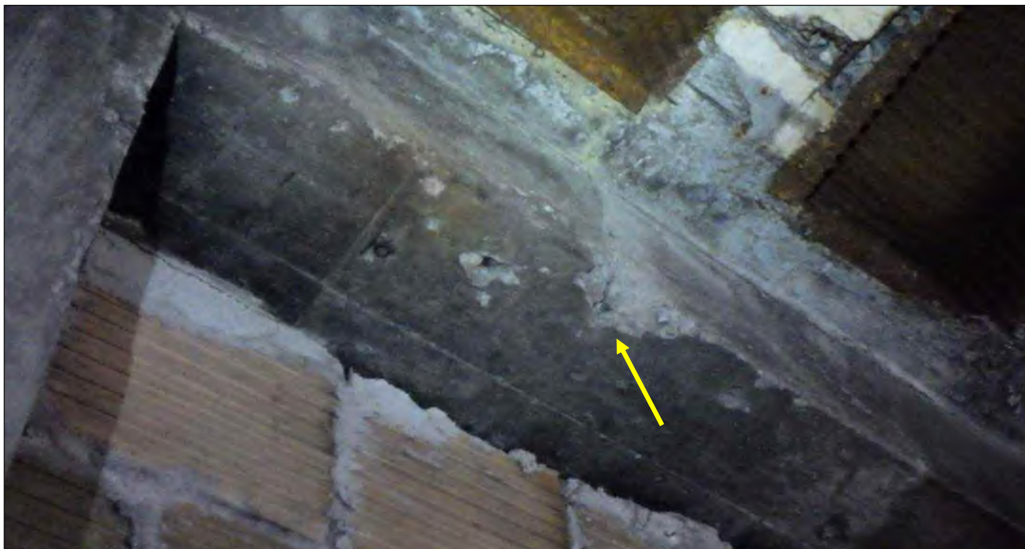
Photo 45: Large missing section of concrete from corner of a beam.
