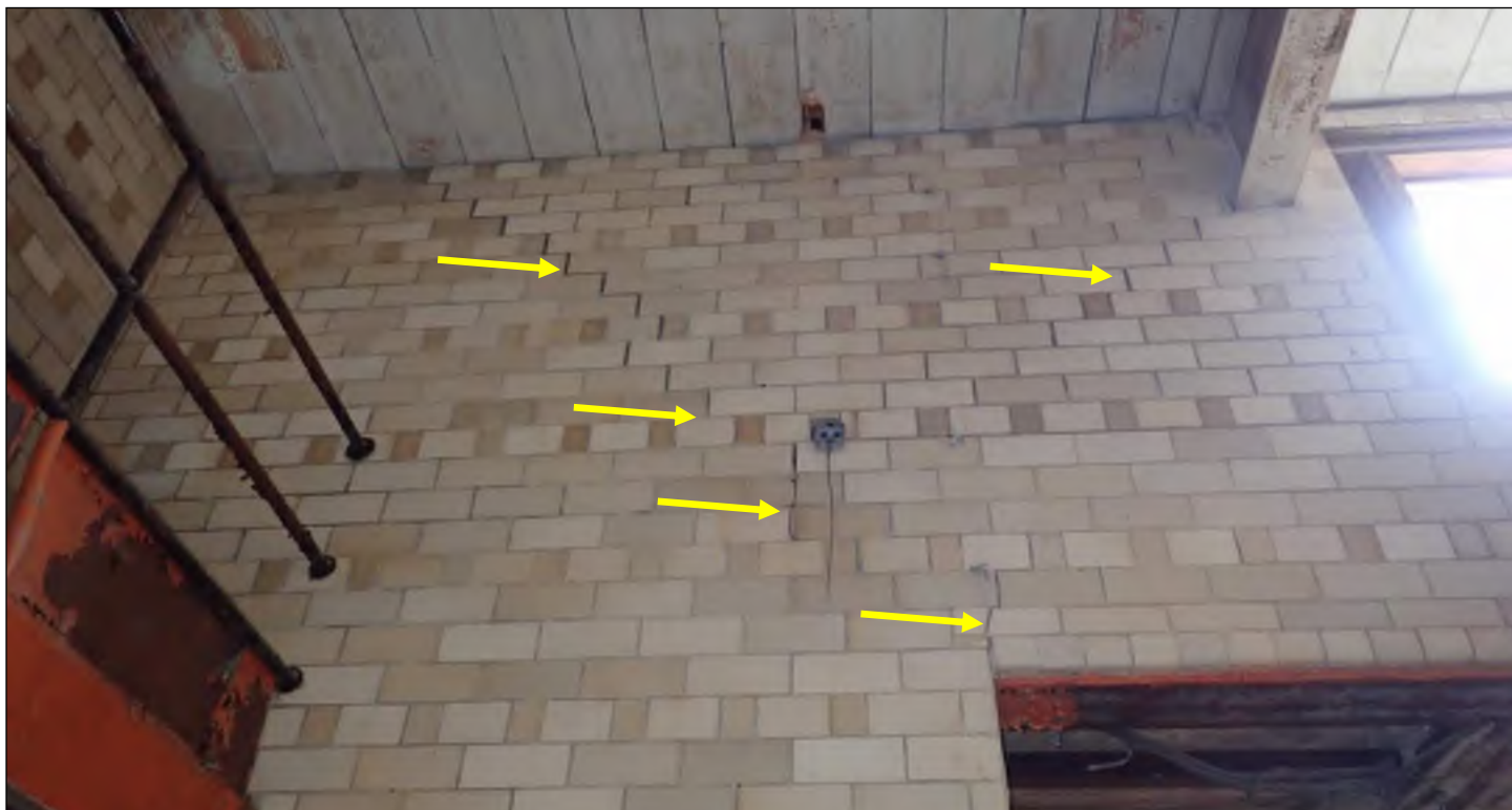
Photo 65: Close-up view of cracking in clay tile finish on west gymnasium wall.
