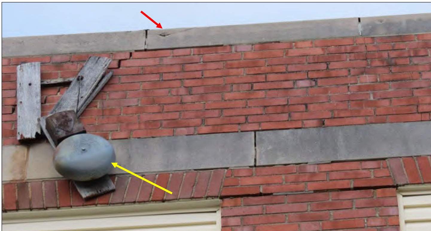
Photo 33: Cracks in parapet coping (red arrow). Note the missing or degraded mortar above and below the limestone band and brick above the windows. Old alarm bell suspended by electrical cable (yellow arrow).
