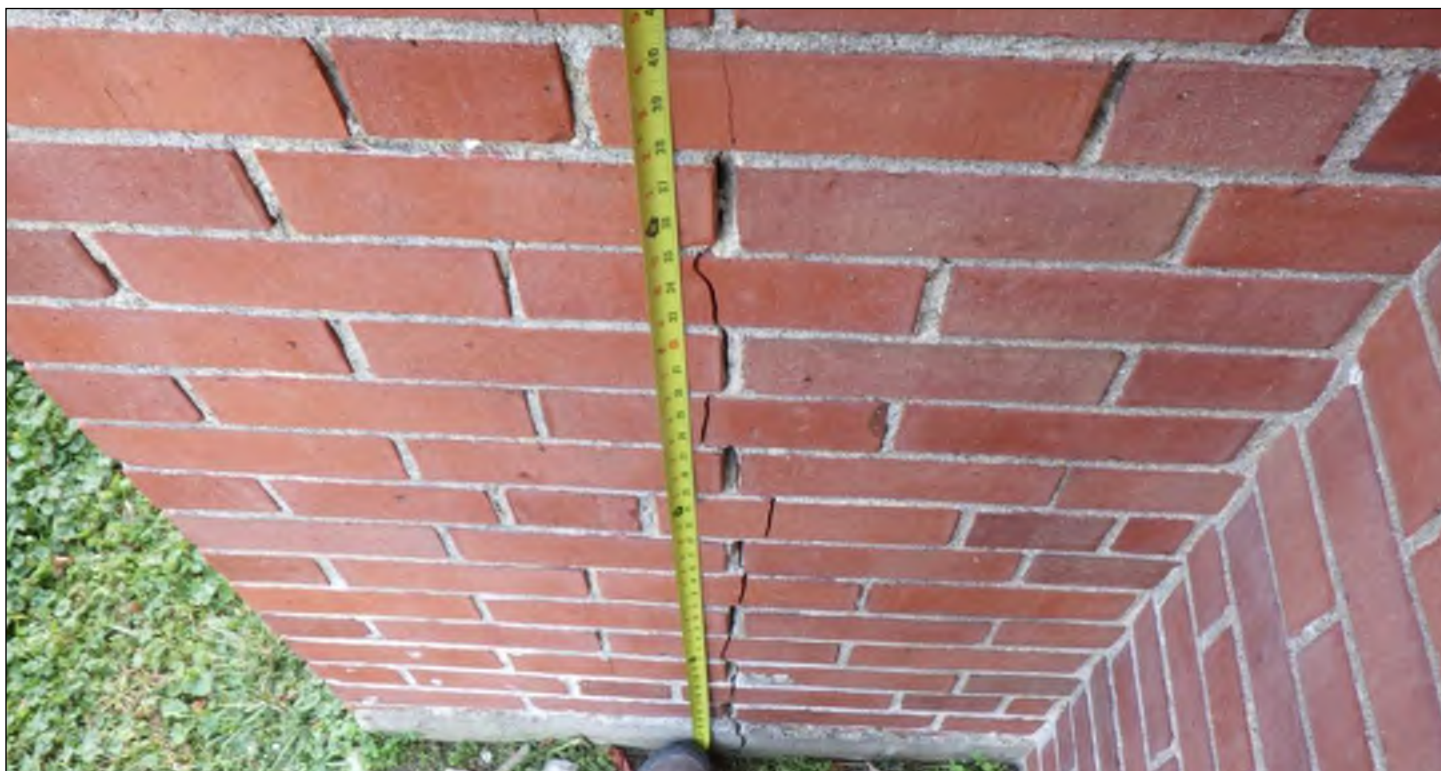
Photo 28: Vertical crack near base of brick masonry bearing wall.
