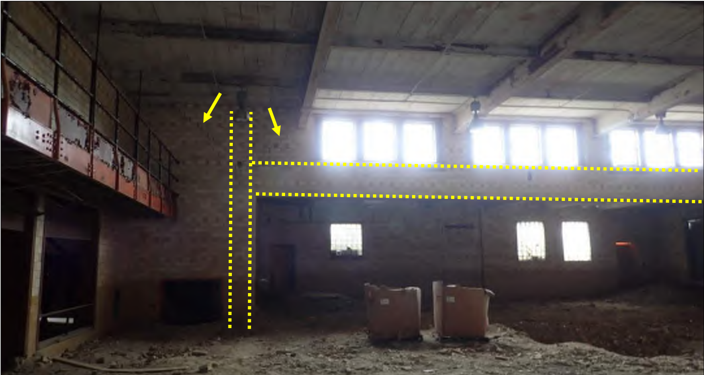
Photo 64: Cracking in clay tile finish on west gymnasium wall (arrows). Note approximate locations of obscured beam and column (dashed lines).
