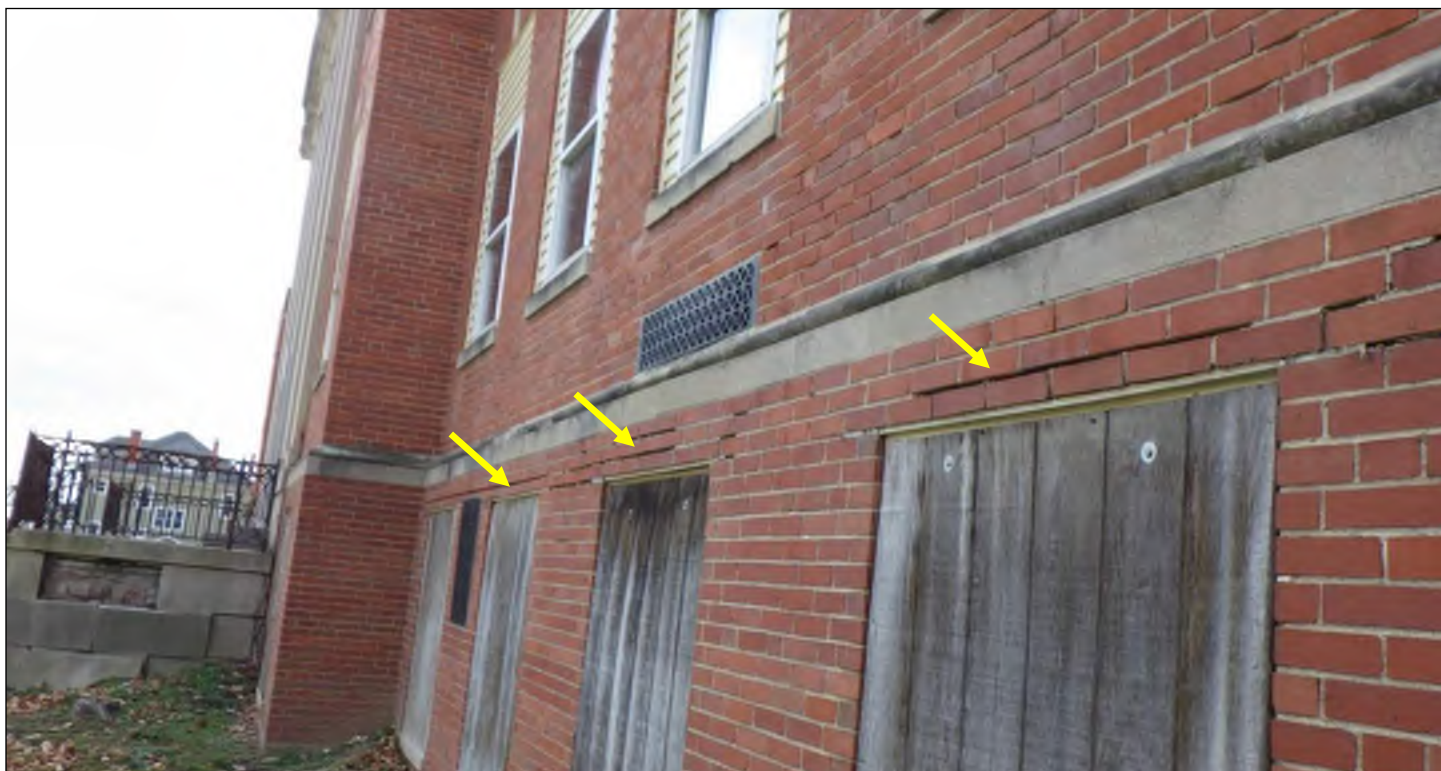
Photo 30: Horizontal cracking and missing or degraded mortar in brick above window openings.
