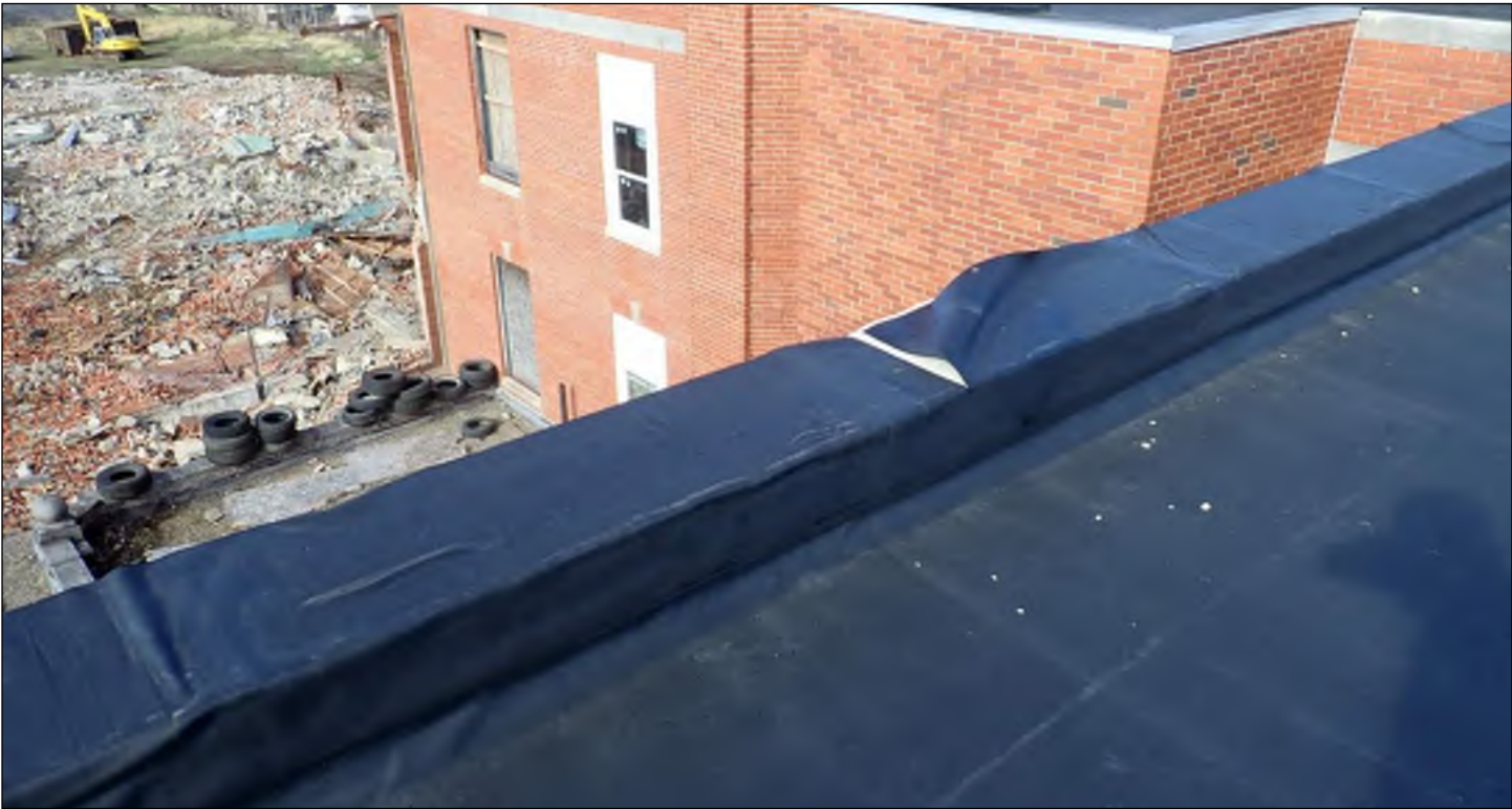
Photo 11: Unsealed roofing membrane.
