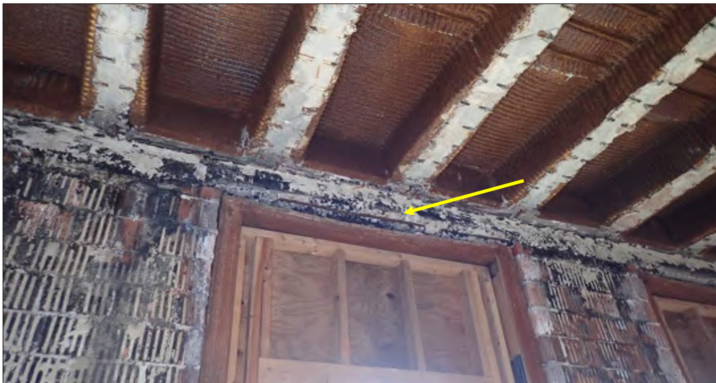
Photo 49: Exposed corroded internal steel reinforcement at a lintel (arrow).
