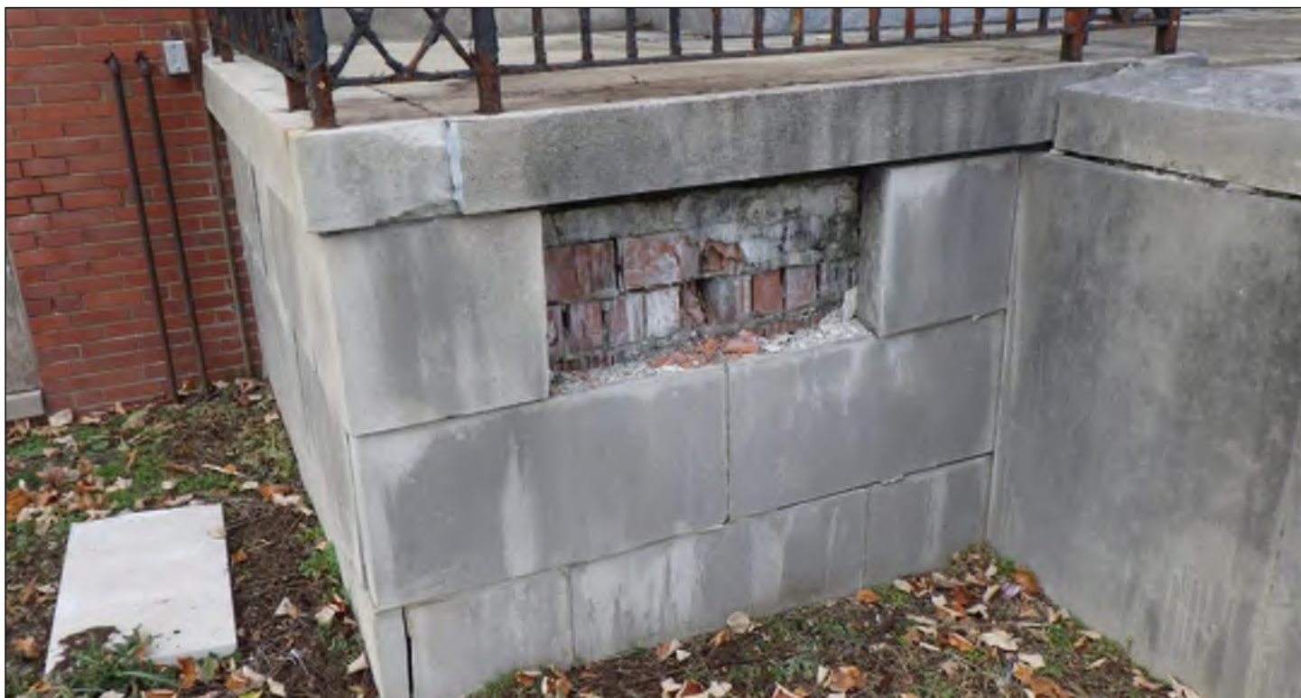
Photo 34: Missing stone block from exterior stairs by east entrance.
