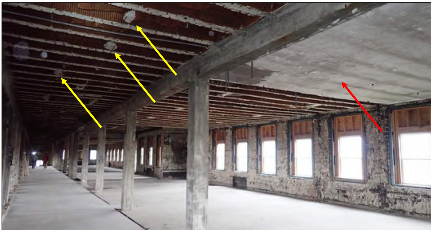
Photo 40: Overall view of reinforced concrete columns, beams, and roof joists with leave-in-place metal tile formwork. Note section of ceiling retaining plaster finish (red arrow) and construction anomalies (yellow arrows).
