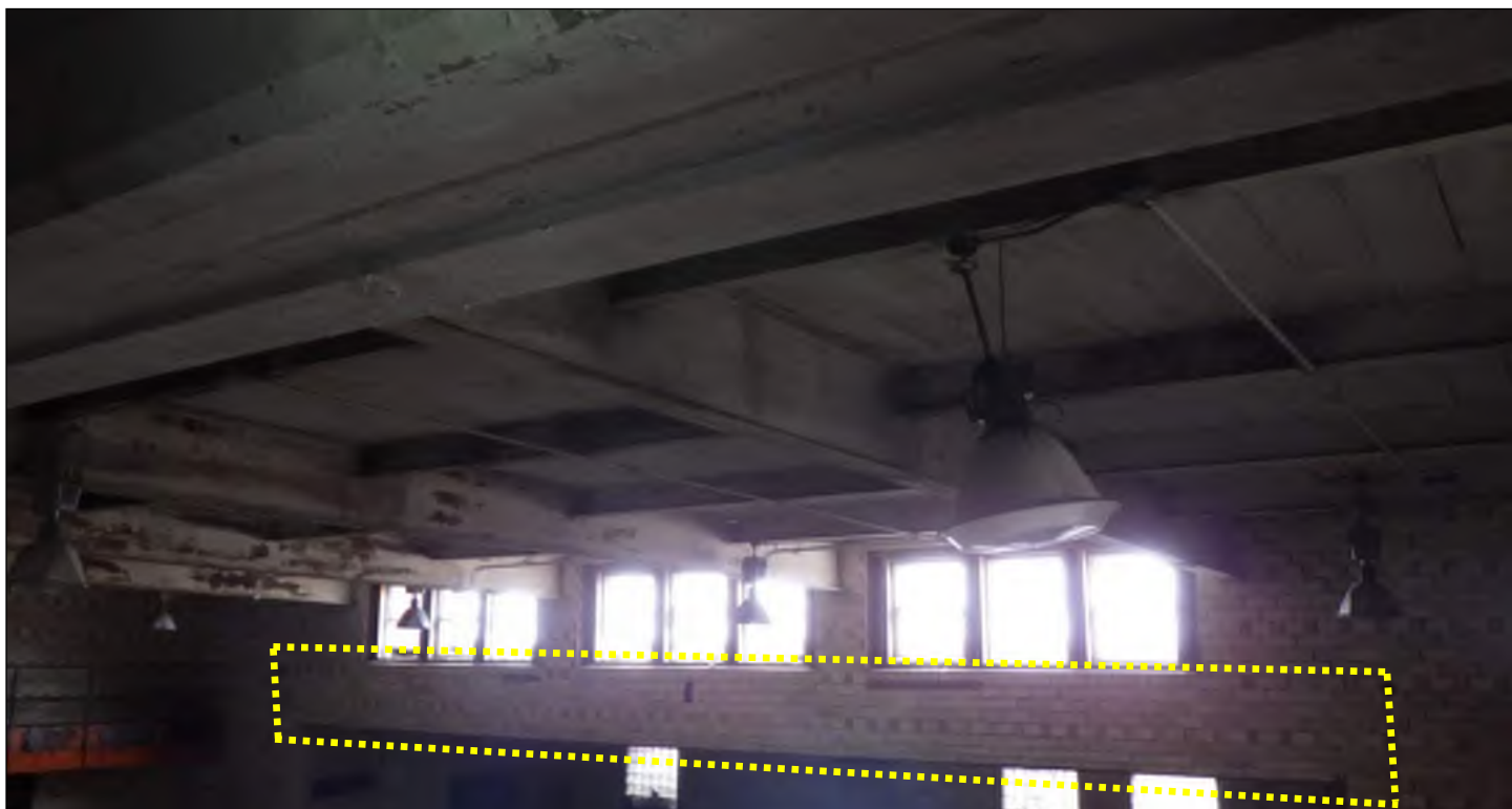
Photo 62: Approximate location of large steel beam at west side of gymnasium (boxed).
