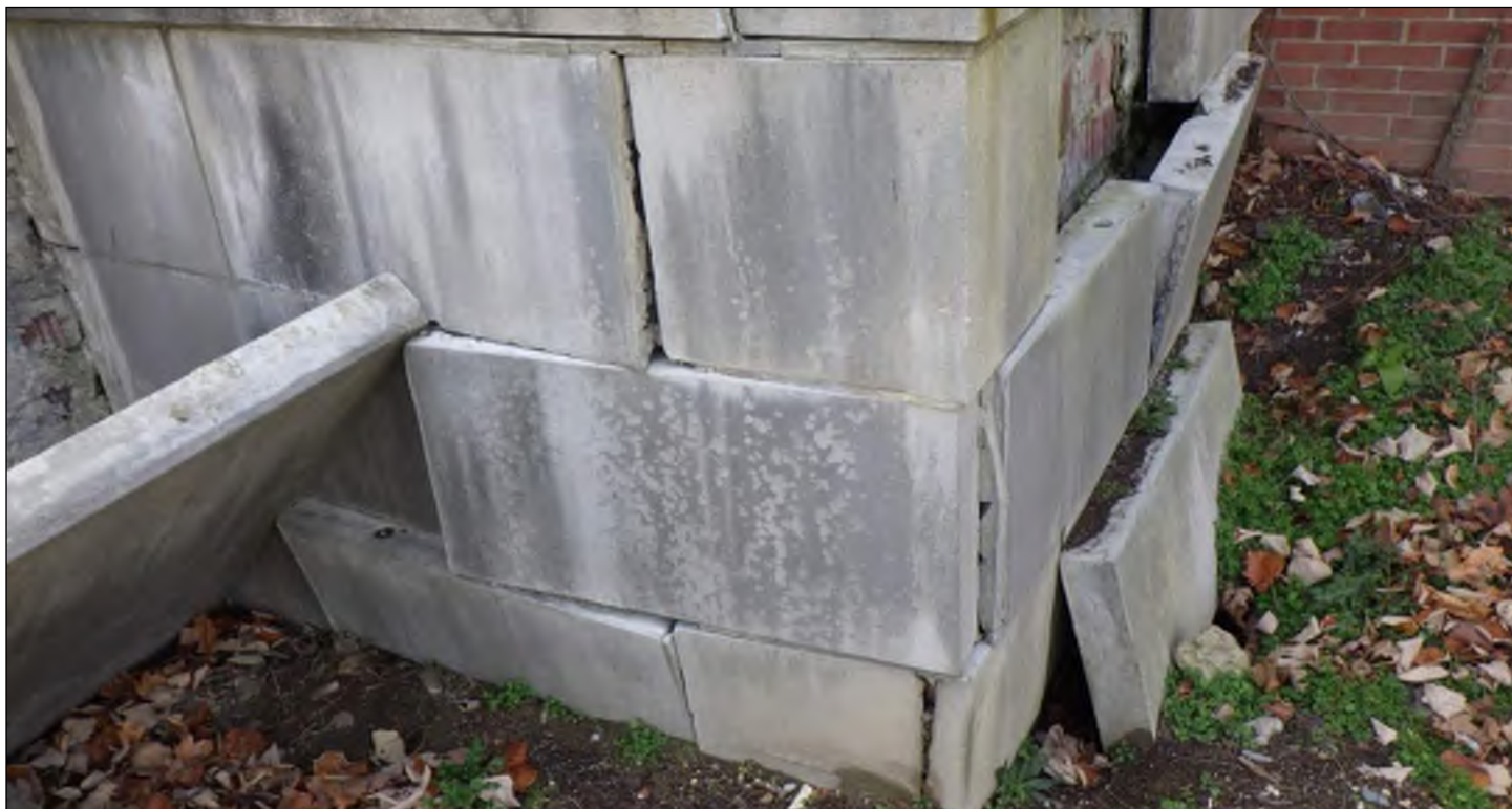
Photo 35: Loose stone blocks at stairs by east entrance.
