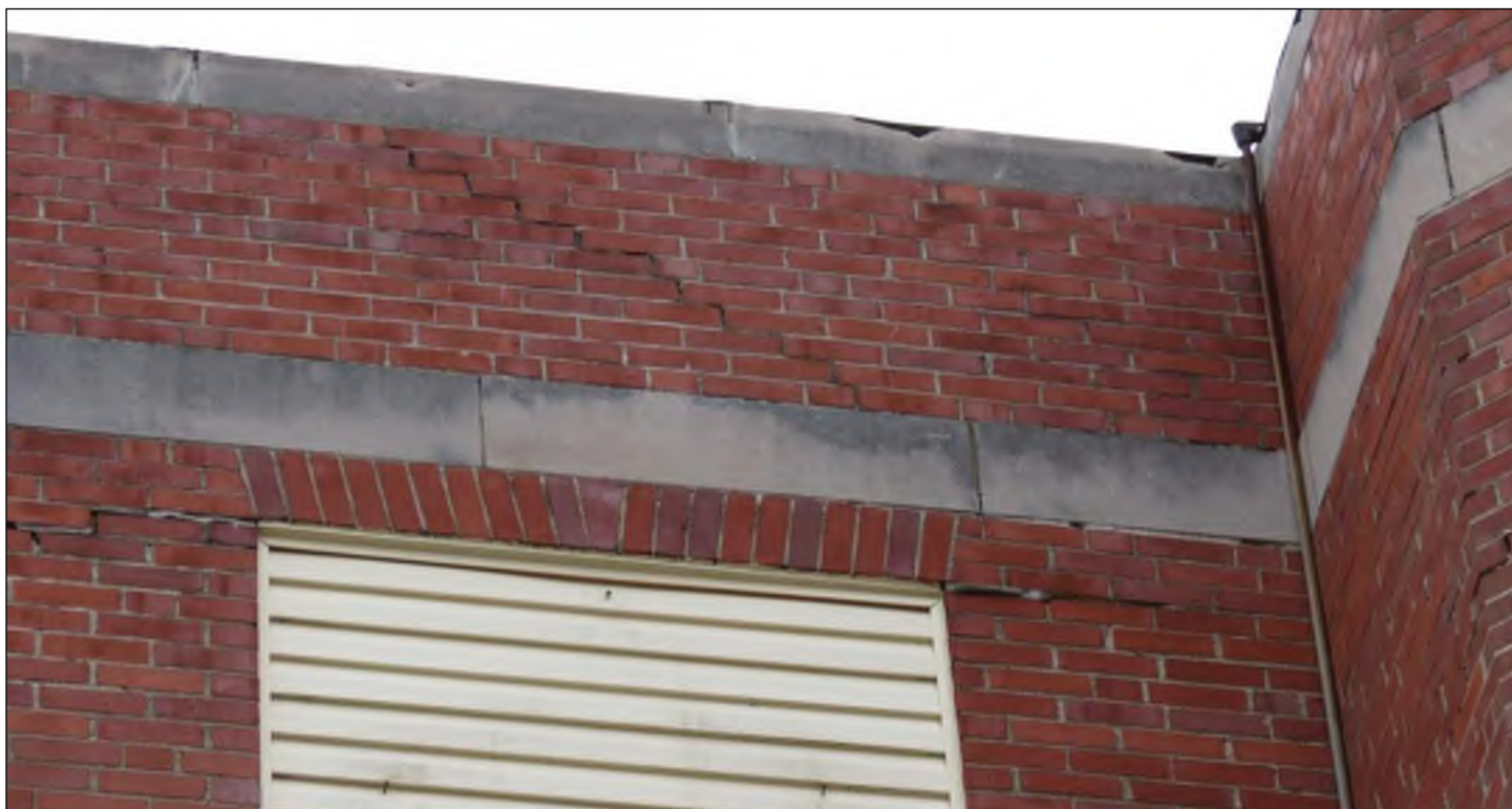
Photo 24: "Stair-step" cracking along parapet mortar joints.
