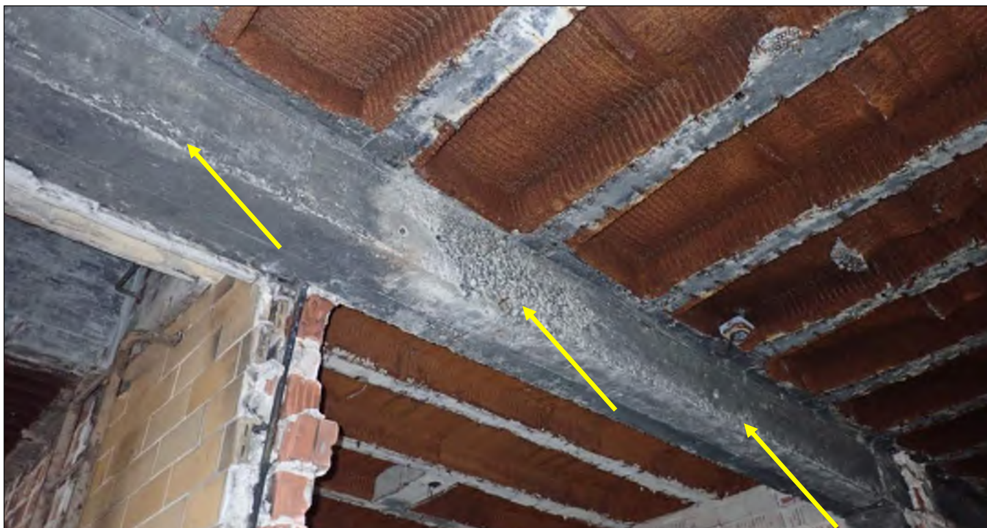
Photo 44: Honeycombing on a reinforced concrete beam (arrows).
