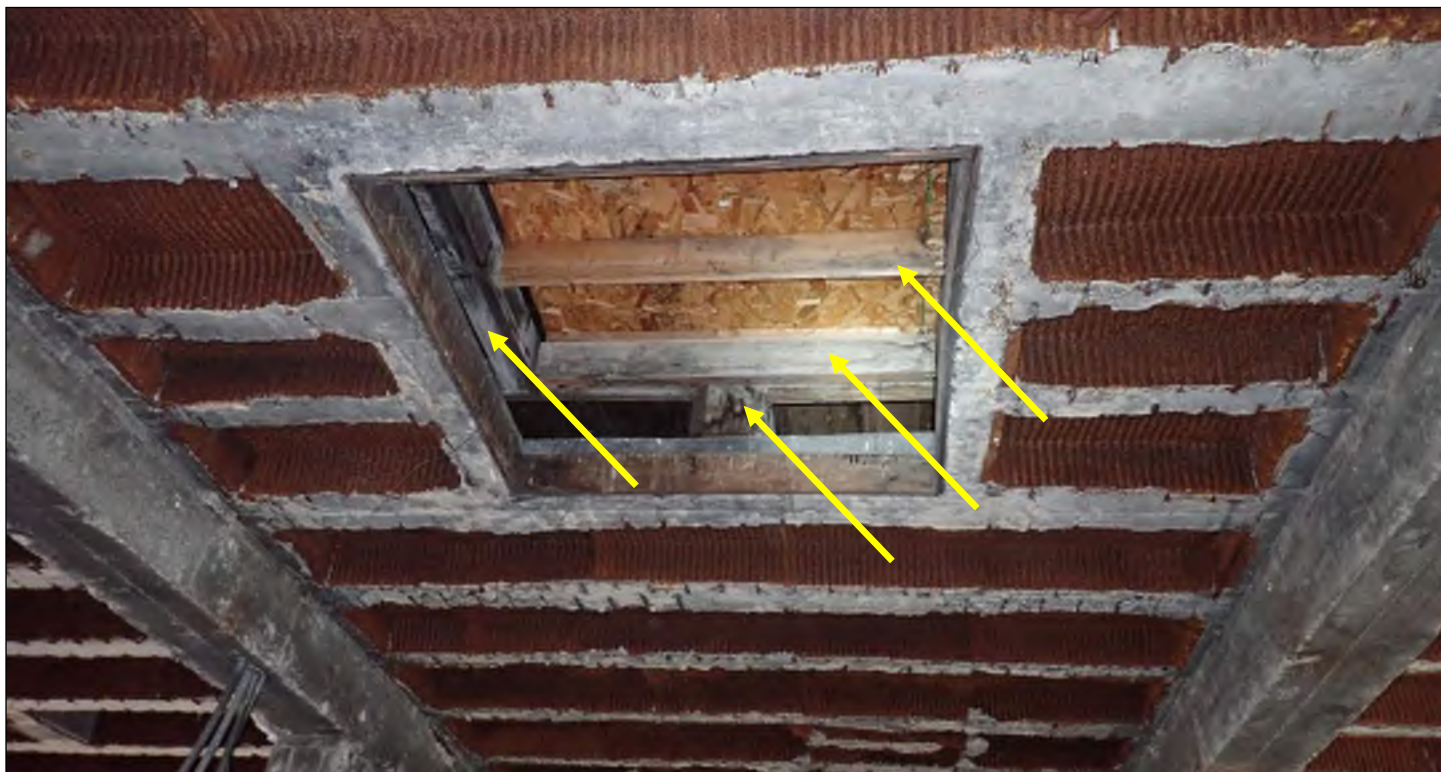
Photo 39: Underside of previous roof addition. Note suspect microbial growth (arrows).
