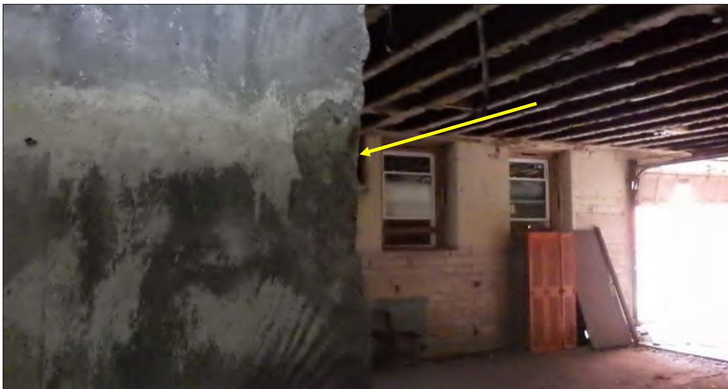
Photo 56: Missing chunk of concrete from the corner of a column (arrow).
