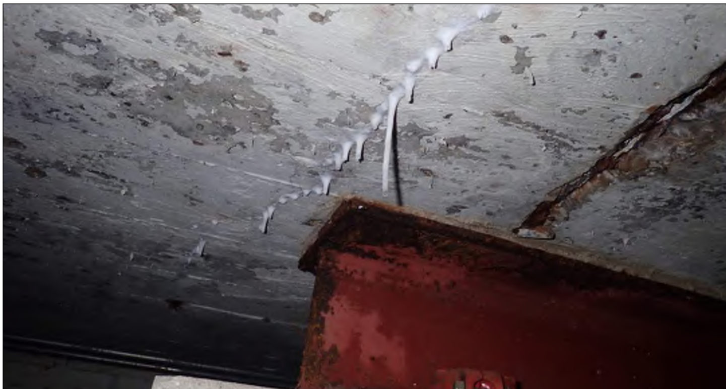
Photo 71: Mineral deposits from water infiltration.
