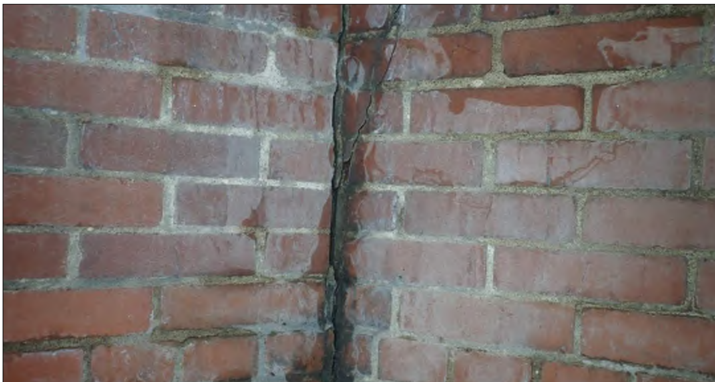
Photo 72: Active water leak at crack in below-grade boiler room wall.
