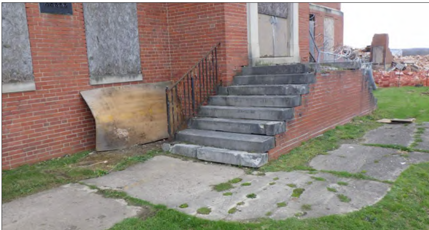
Photo 38: Exterior stairs by north entrance. Note the lack of finished walking surface and handrails.
