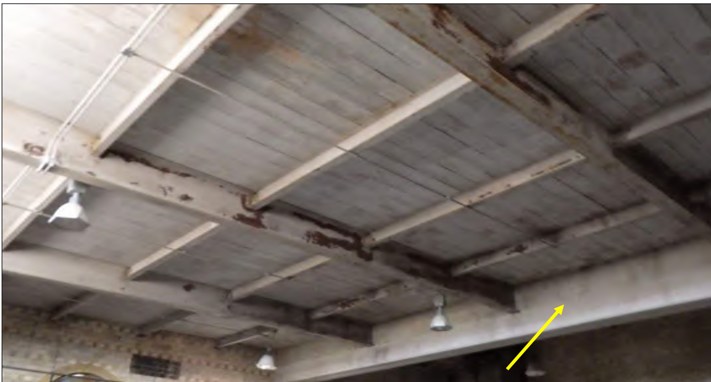
Photo 59: Overall view of steel beams supporting the gymnasium roof, looking north. Note the steel plate girder at the east side of the roof (arrow).
