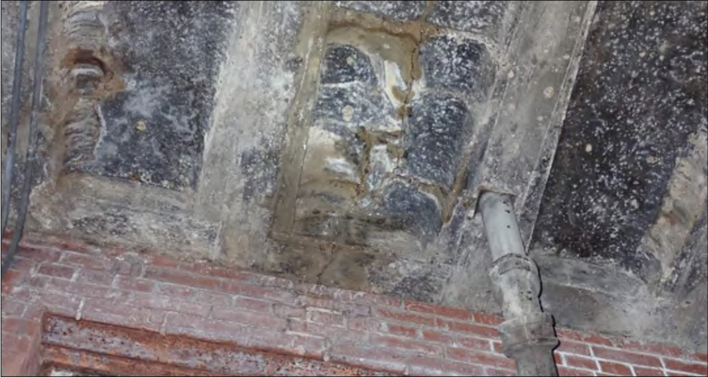
Photo 69: Cracking and water staining at the underside of the boiler room roof slab.
