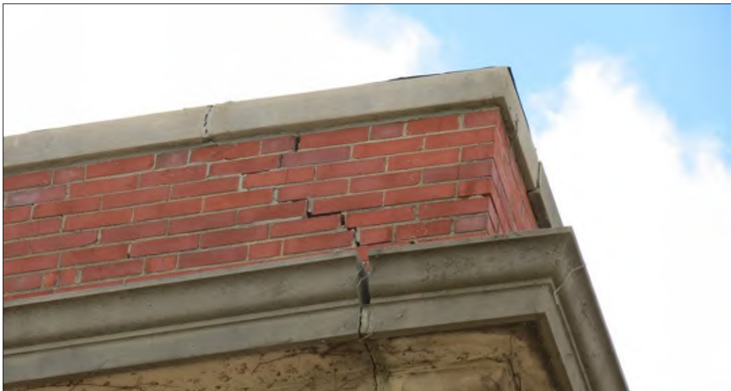
Photo 23: Cracking near parapet corner.
