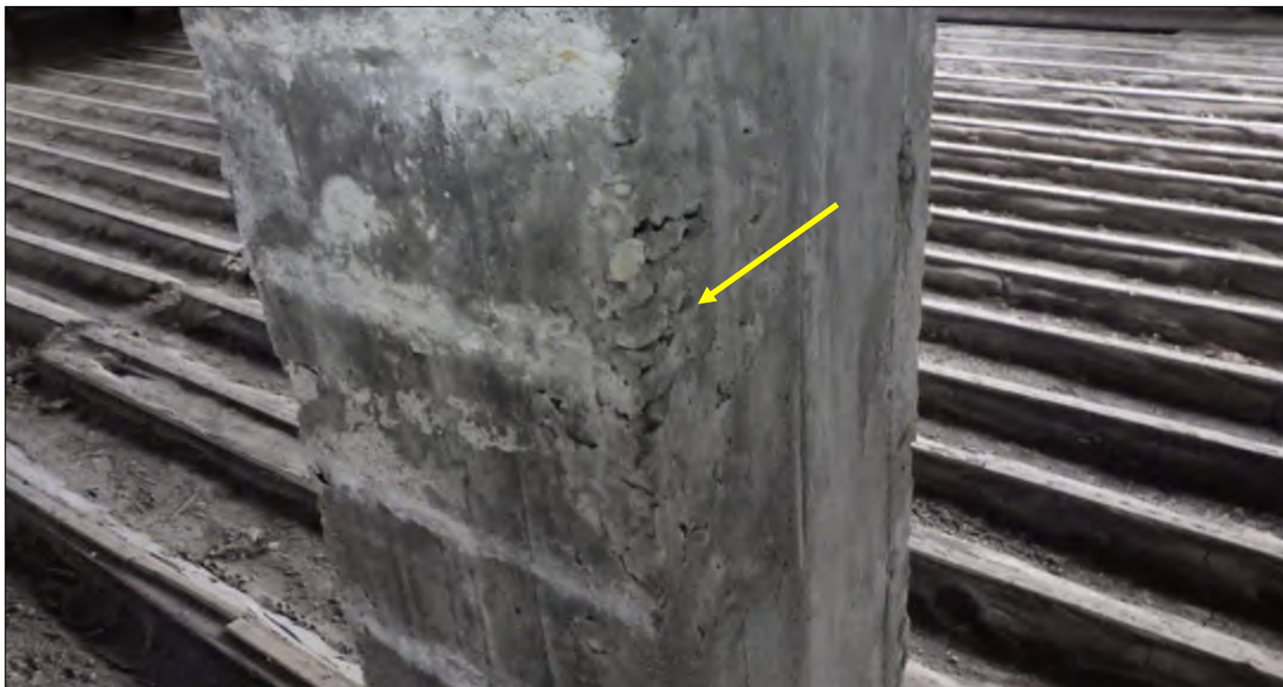
Photo 55: Honeycombing on a reinforced concrete column (arrow).
