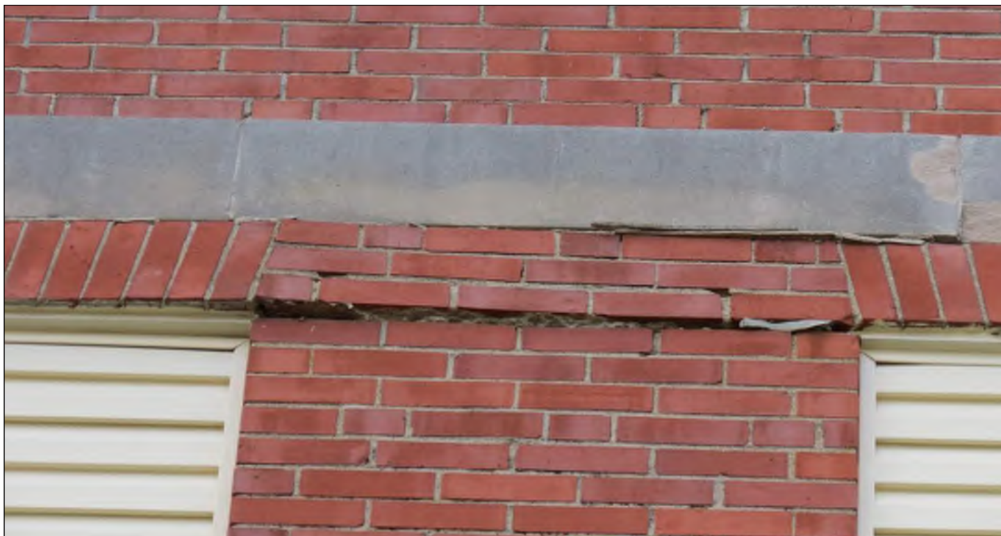
Photo 31: Horizontal cracking and missing or degraded mortar in brick above window openings.
