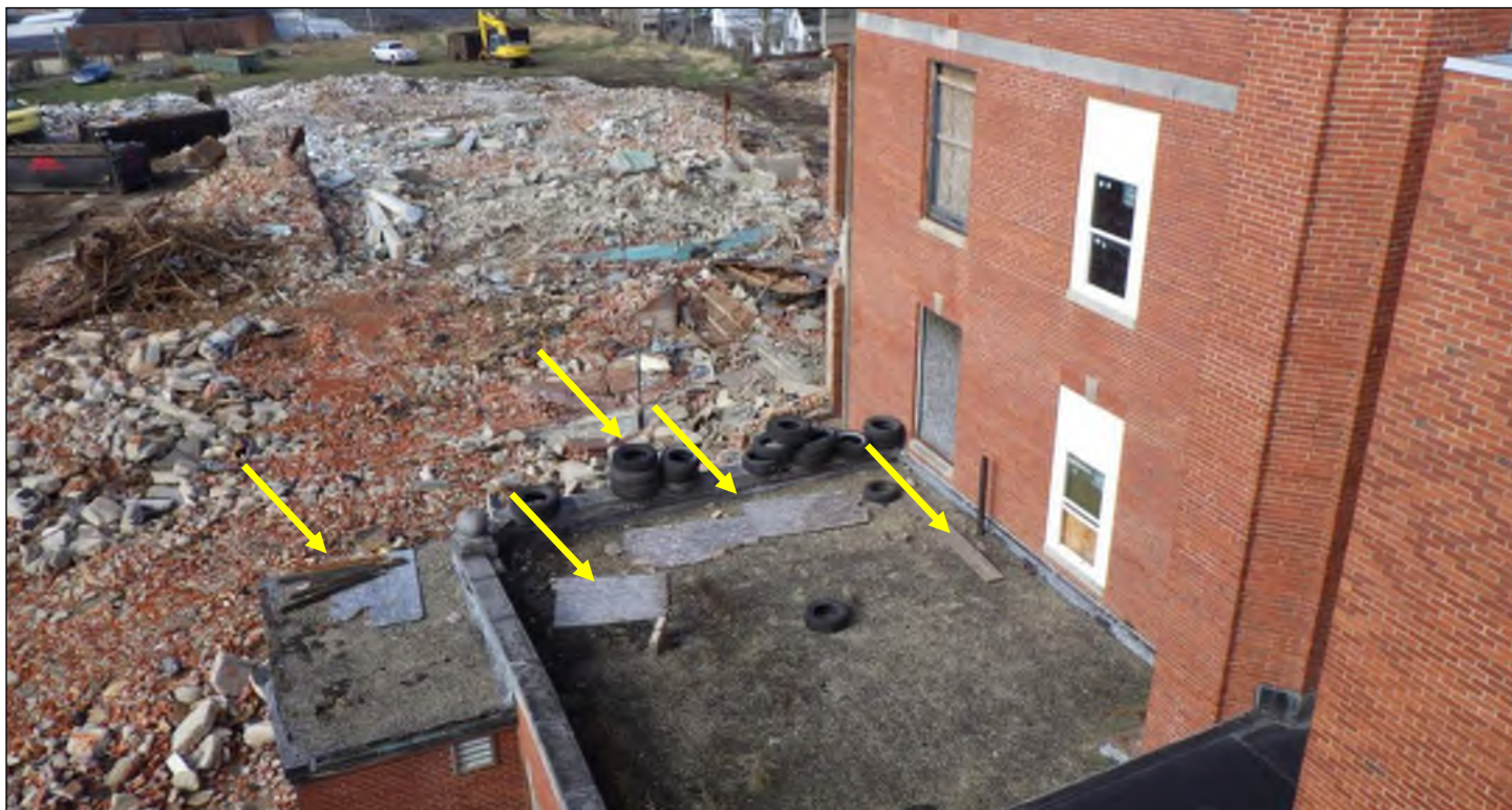
Photo 15: Overall view of boiler room roof, looking west. Note debris apparently from demolition of adjacent structure (arrows).
