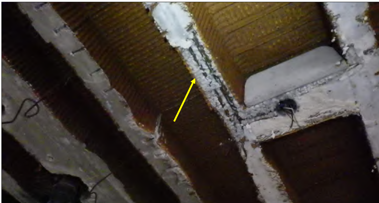
Photo 47: Exposed corroded internal steel reinforcement at a joist (arrow).
