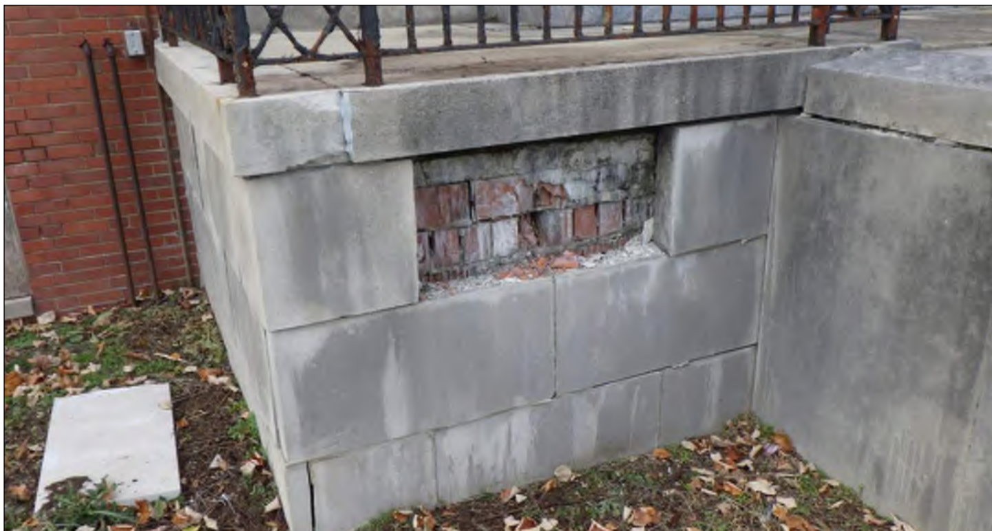
Photo 37: Cracked/spalled bricks at exterior stairs by east entrance.
