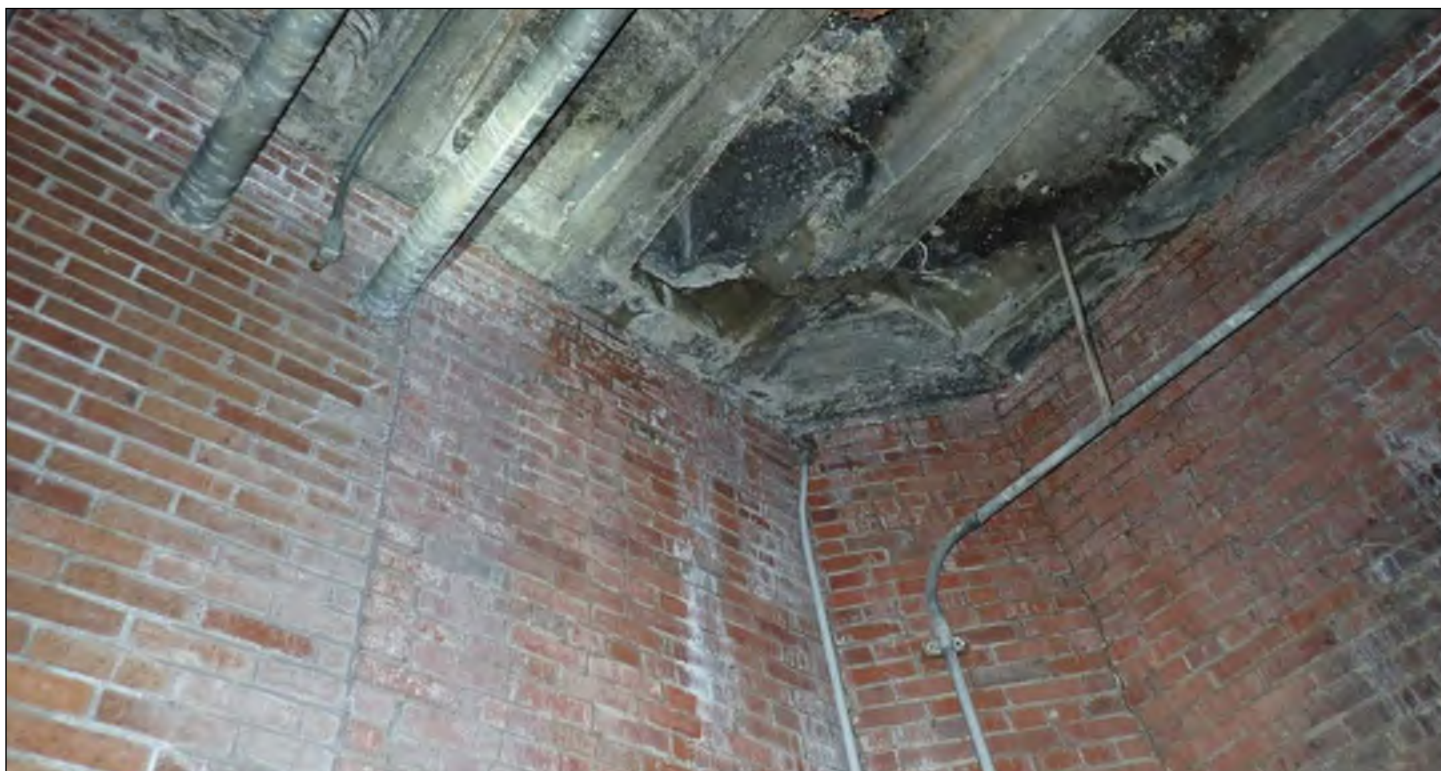
Photo 68: Cracking and water staining at the underside of the boiler room roof slab.
