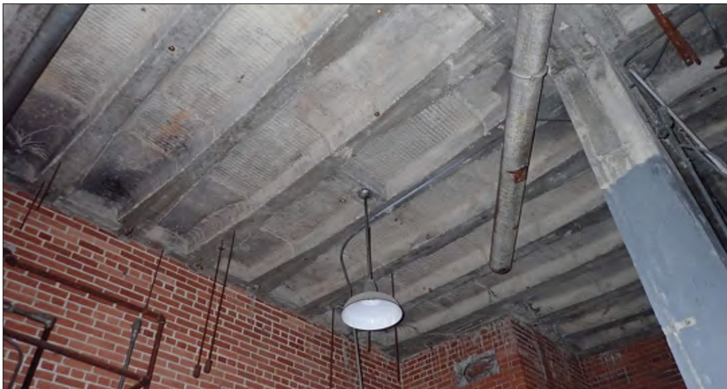
Photo 67: Underside of boiler room roof slab. Note the lack of metal tile formwork.
