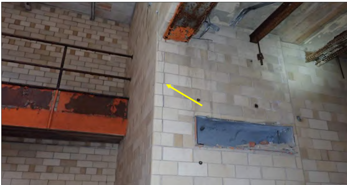
Photo 66: Close-up view of cracking in clay tile finish on west gymnasium wall.
