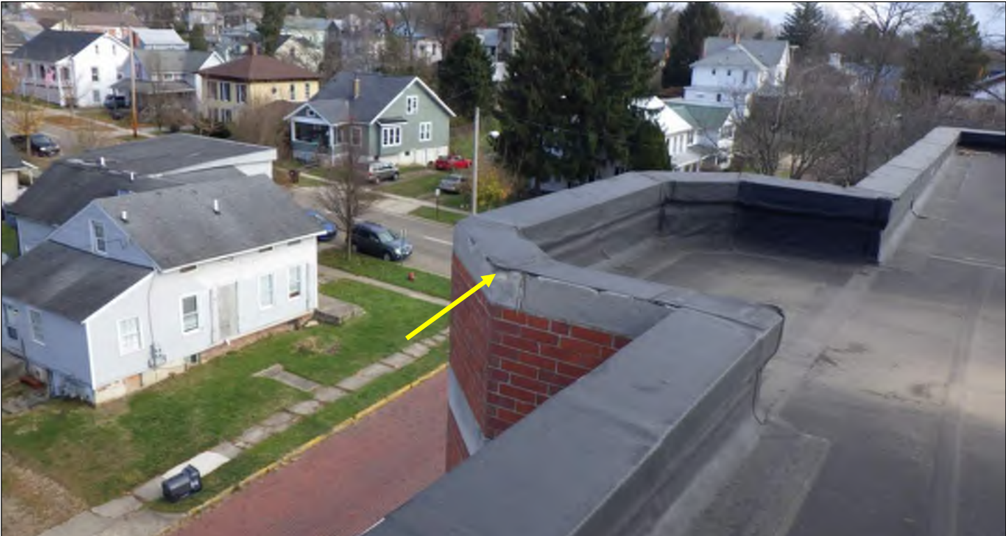
Photo 22: Old spalls on parapet, with dirt buildup on surface.
