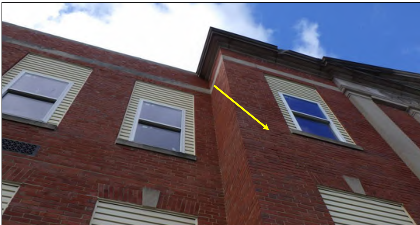
Photo 26: Crack propagating from corner of window opening.
