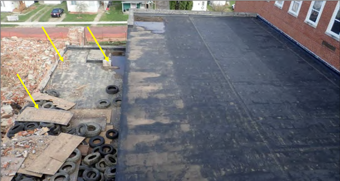
Photo 12: Overall view of high and low gymnasium roofs, looking north. Note dirt and debris apparently from demolition of adjacent structure (arrows).
